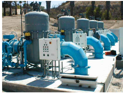
Five 24" Eaton Model 2596 strainers with backwash assist pumps installed at a potable water treatment plant.
